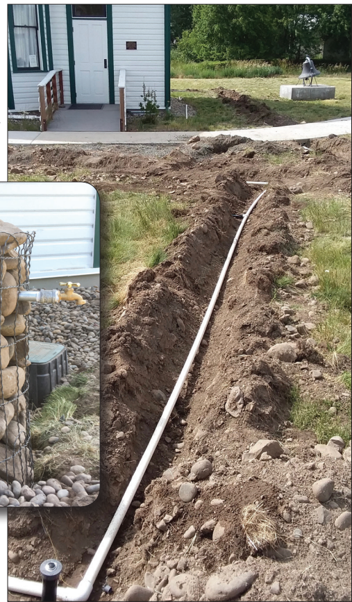
Left: John Hutchens glues pipe. Center: A "rock-post" supports a faucet. Right: Rocks present a challenge.
